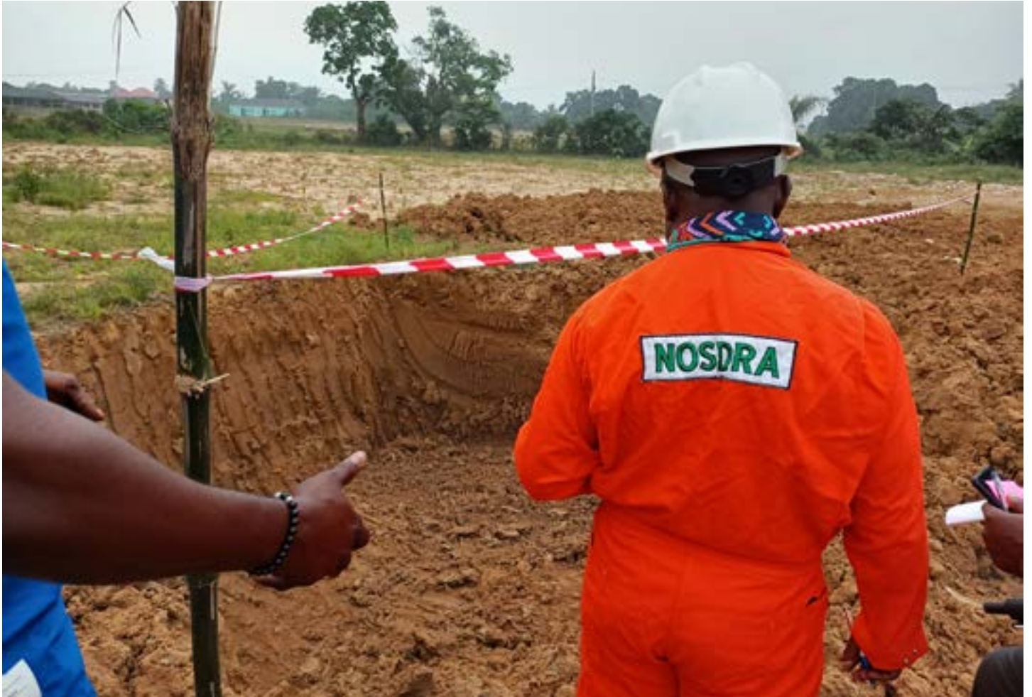
Excavation pit inspection at Lot 42 in Korokoro community in Tai Local Government Area
